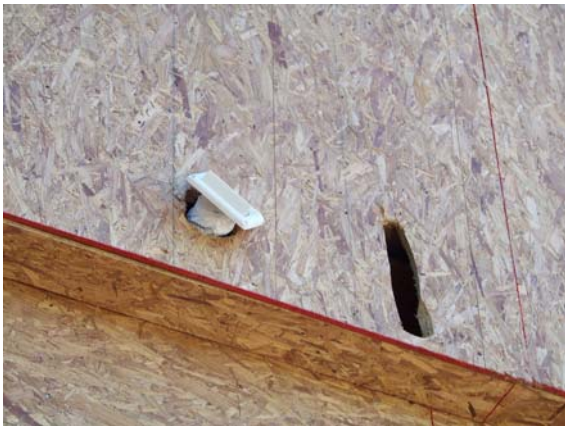
Un-sealed openings in OSB sheathing
