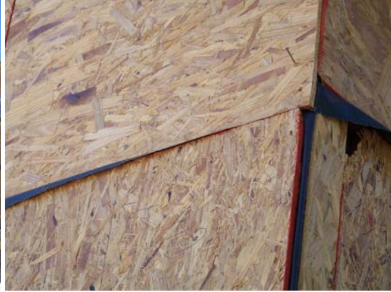
Flashing not present between sheets
