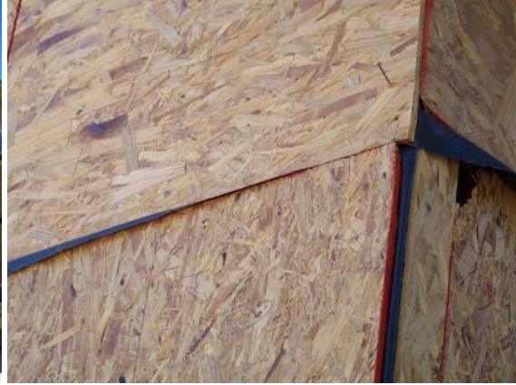
Flashing not present between sheets
